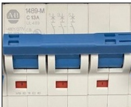
Bank 1 Breaker Closed/Hot
