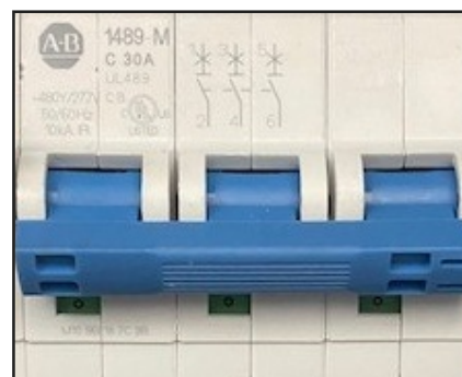
Bank 1 Breaker Open/Tripped
