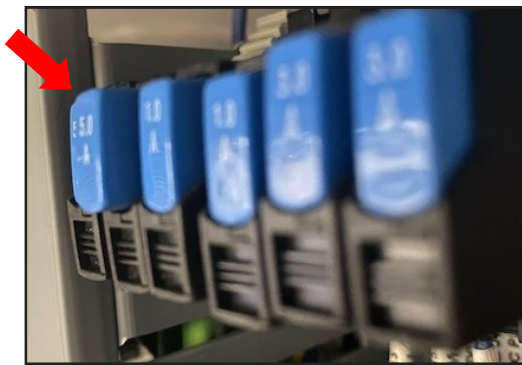
Bank 3 Breaker Tripped
