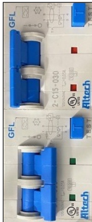
Bank 3 Breaker Closed/Hot (ON)
